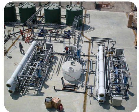
RO Installation at Michilla
